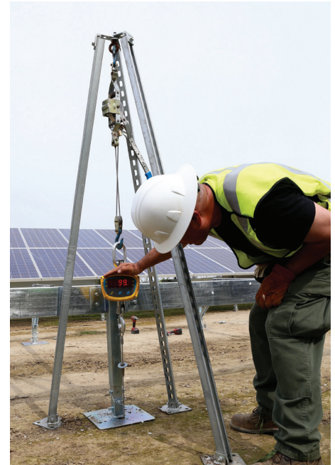
The holding strength of an earth anchor being verified in real-time during the installation of an Osprey PowerPlatform. Photo Courtesy of Nuance Energy.
